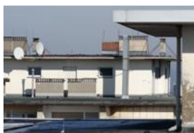
Power cable on the roof
