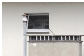
Power cable reaching the socket
